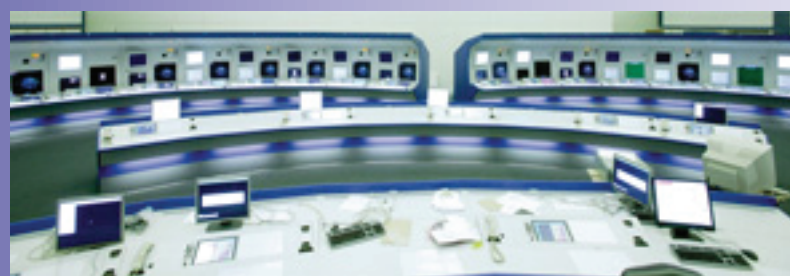
Control Room Workstations
