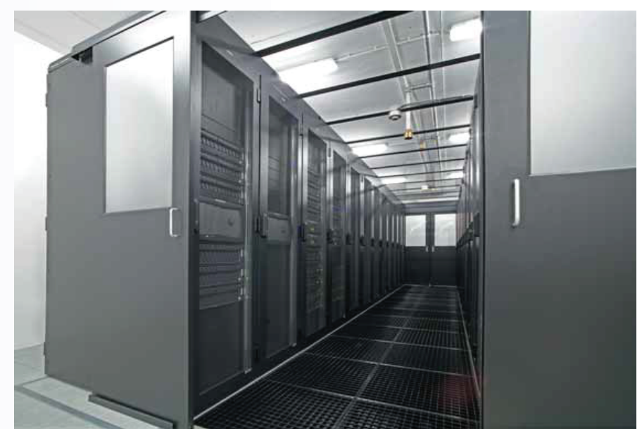
Data Center Solutions
